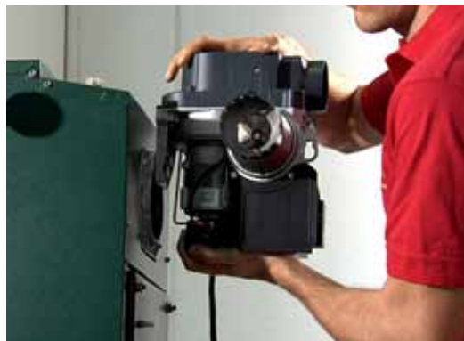
Dedicated Servicing Position.
